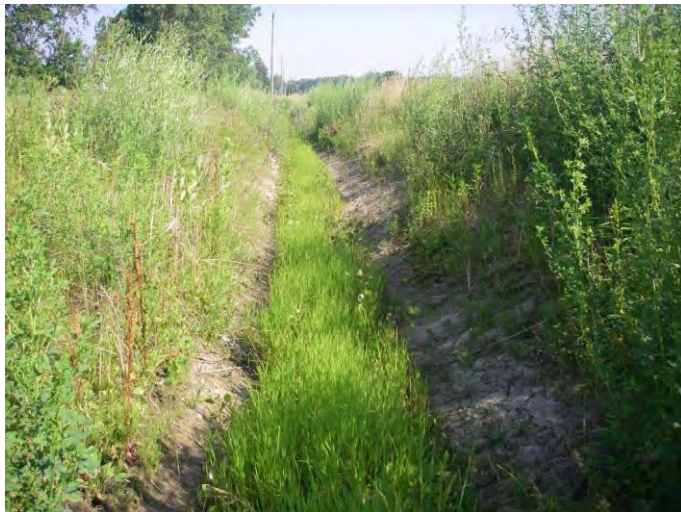
Photo 29: Station 73-2 – East Kelly Drain (Summer 2012) - Facing upstream (west) from Dunnville/Wainfleet Townline, showing dredged ditch.
