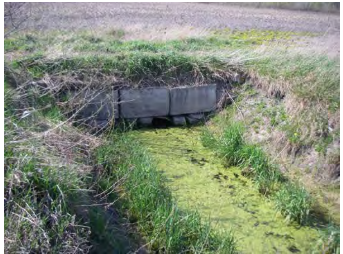
Photo 8: Station R11T072-1 – Unnamed Tributary to Upper Welland River (Summer 2012) - Facing downstream (south) east of Gore Road, showing channel and culvert.
