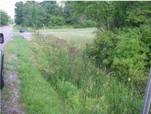
Photo 33 Station 55-1 – Fifteen Mile Creek (Summer 2012) - Facing upstream (west) from Concession 4, showing channel overview along roadside.
