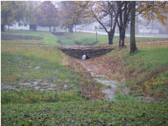
Photo 51: Station 15-4 - Mill Race Creek (Fall 2012) - Facing downstream (east) from Canal Bank Road, showing channel and surrounding manicured lawn.
