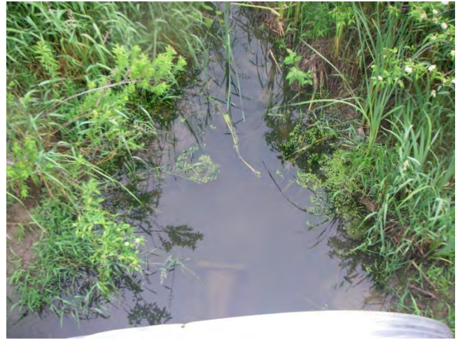
Photo 38: Station R11T099-2-Tweed Drain (Summer 2012) – Off of Inman Road, showing close up of channel from culvert.
