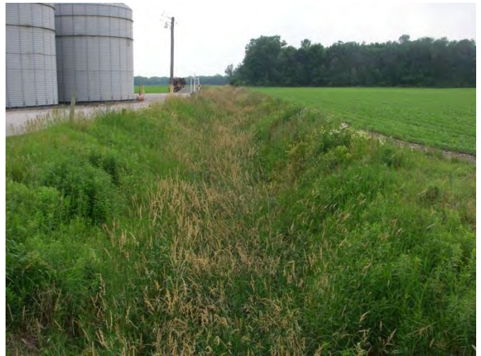
Photo 8: Station 71-1 – Ellsworth Drain (Summer 2012) - Facing upstream (west) from Hendershot Road, showing channel overview.
