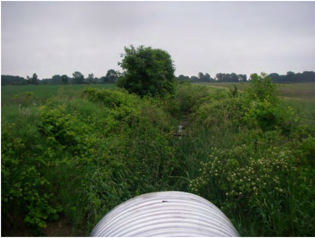
Photo 37: Station R11T099-2-Tweed Drain (Summer 2012) – Facing downstream (east) off of Inman Road, showing channel overview.
