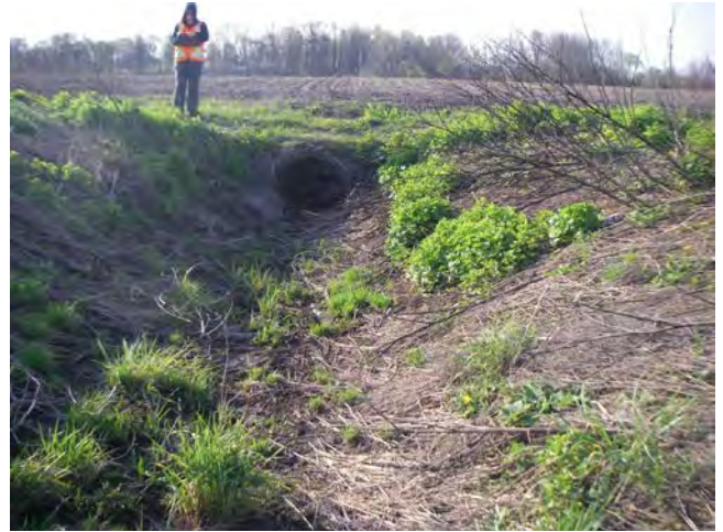
Photo 14: Station R11T082-2 – North Forks Drain (Summer 2012) - Facing downstream (south) east of Gee Road, showing channel overview.
