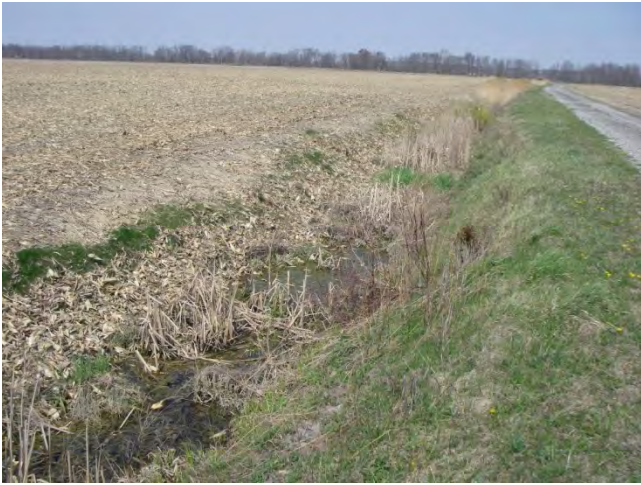
Photo 13: Station R11T045-2 –Broad Creek Drain (Summer 2012) - Facing upstream (north) south of Canal Bank Road, showing channel overview alongside road.
