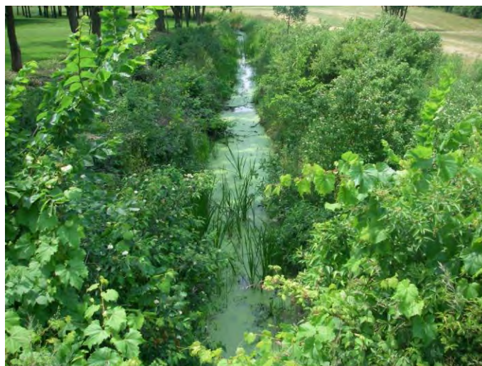
Photo 4: Station 65-4 – North Forks Drain (Summer 2012) - Facing downstream (east) from Shafley Road, showing channel overview and instream vegetation.
