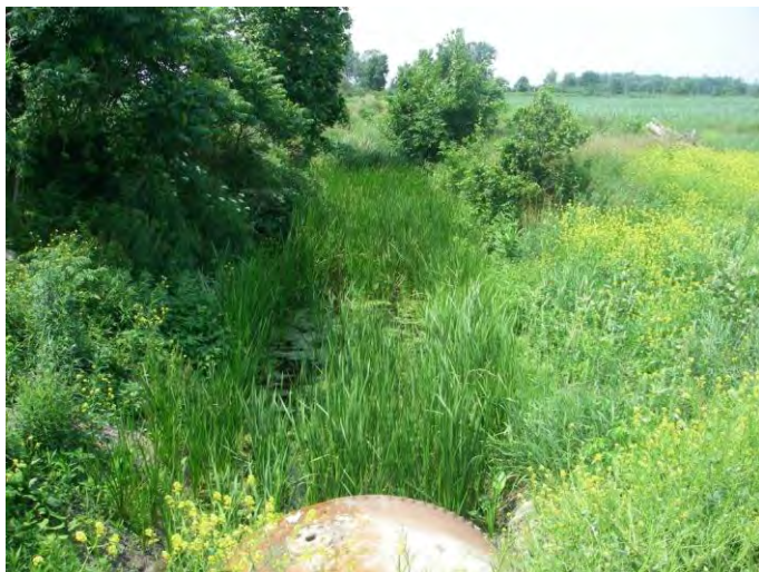
Photo 1: Station 65-3 – Wolf Creek Drain (Summer 2012) - Facing upstream (northwest) from Shafley Road, showing channel overview from culvert.
