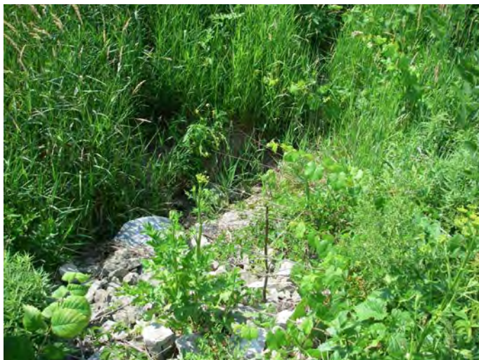
Photo 9: Station 31 -1 – Tributary to the Welland River (Summer 2012) - Facing upstream (southeast) from Creek Road, showing culvert leading into agricultural swale.
